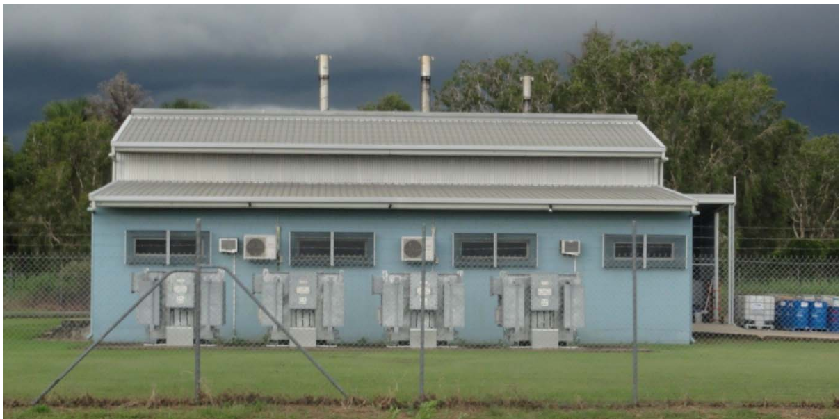
Image 12 – Our town's power generator
