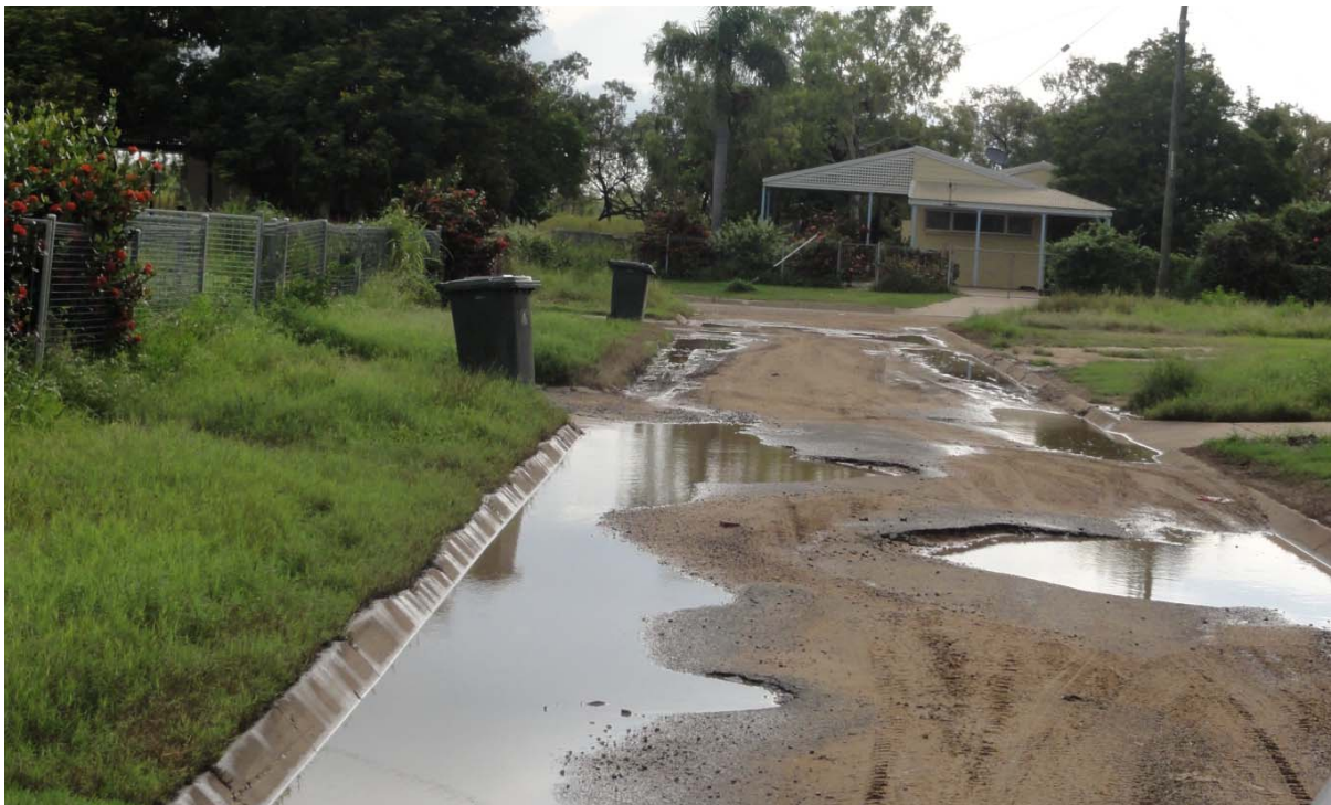
Image 11 – An example of a road that needs fixing because of bad stormwater drainage
